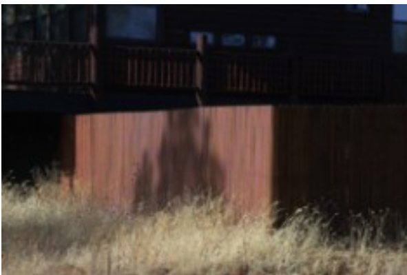
No 1 inch spacing between slats.
